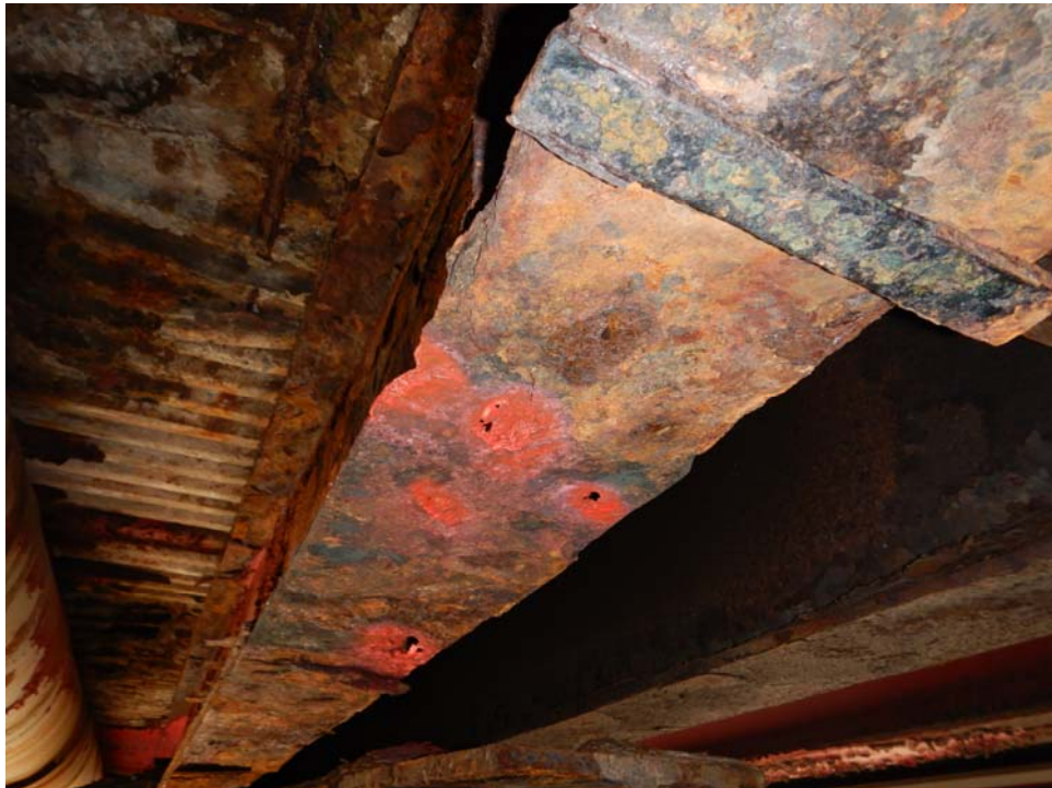
Beam 11 at far \frac{1}{4} point, looking back. Note flange holes and section loss.
