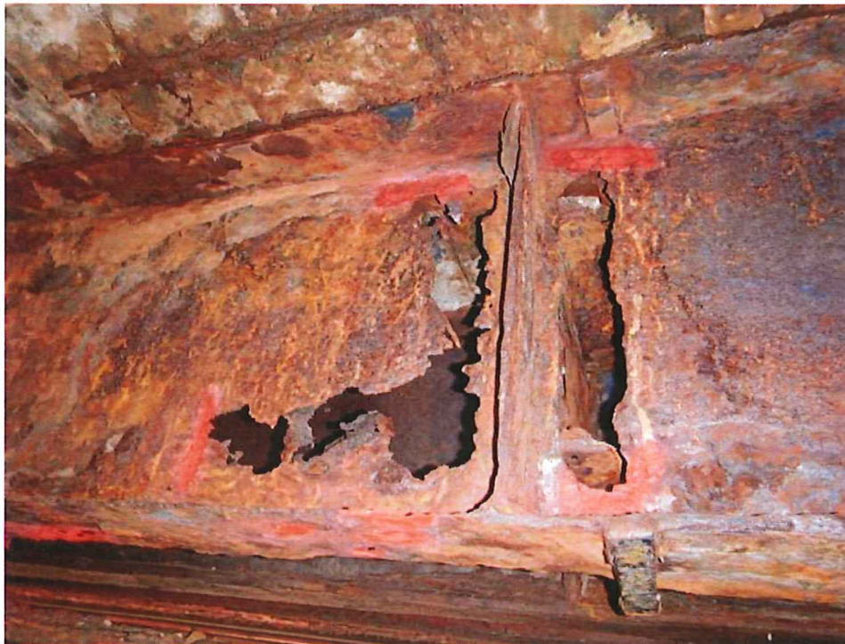
Beam 11 at far \frac{1}{4} point, looking left. Note web holes.
