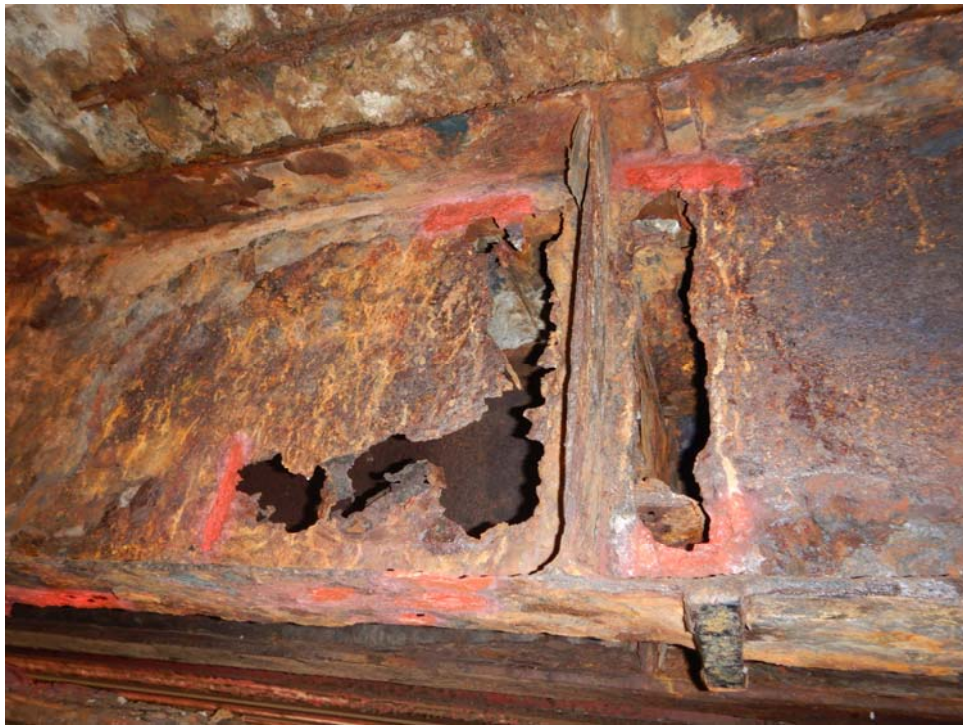
Beam 11 at far \frac{1}{4} point, looking left. Note web holes.
