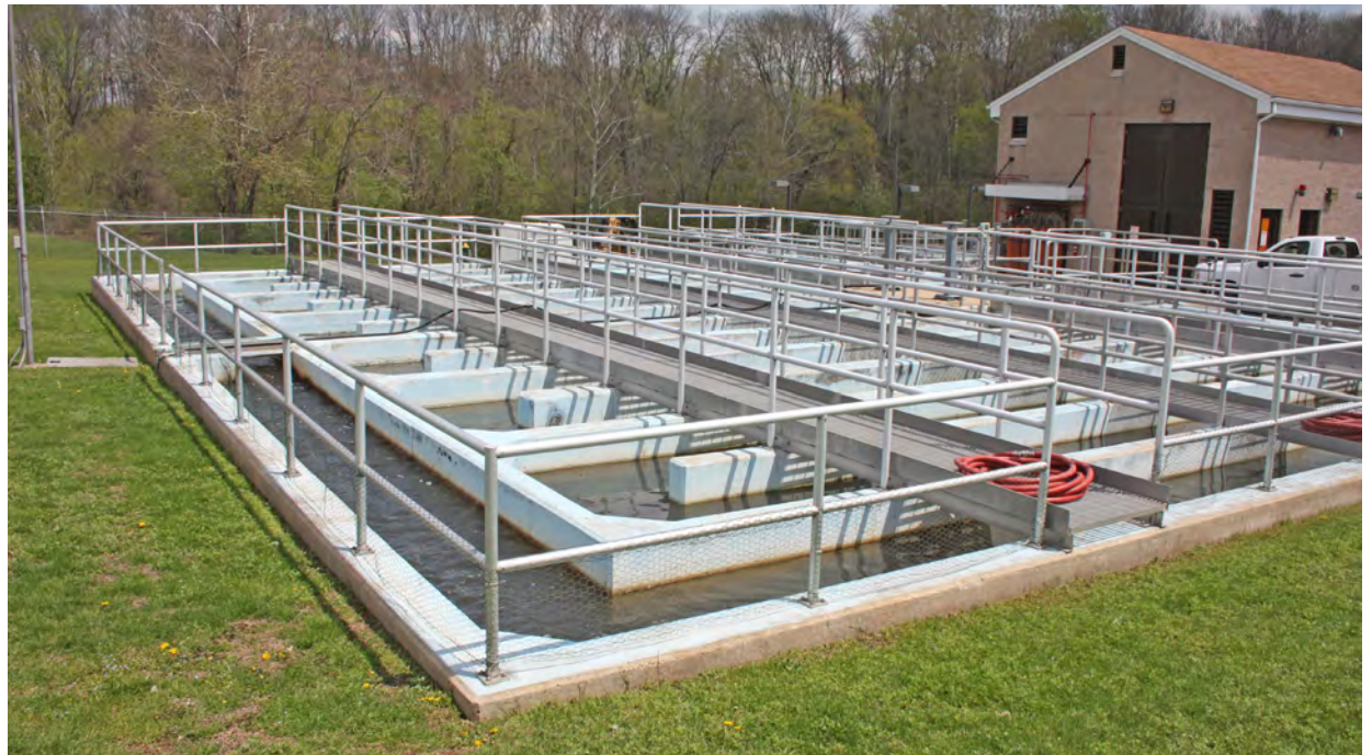
Trout Run Treatment Plant
